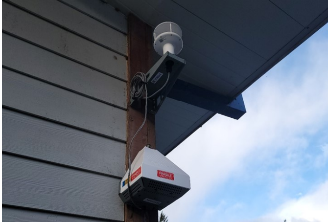
AQMesh Pod for the DEC Community-Based Air Monitoring Project
